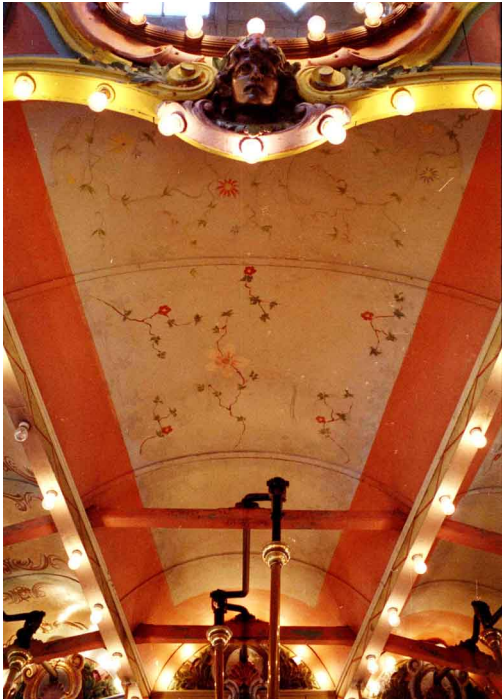
The ceiling panels had been overpainted with scattered flowers and orange borders.
